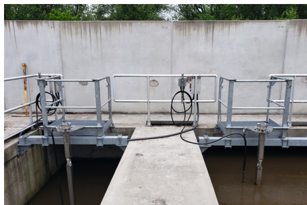
Landia mixer guide rails at Milton
